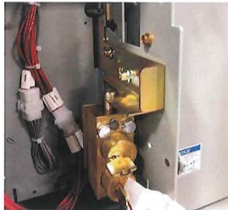
Figure 6 – External Key Interlocks
